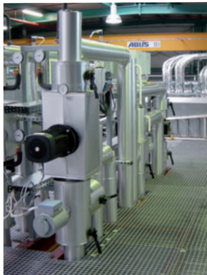
Pump stations for conditioning system
